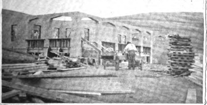
Completing the first floor of the Assistant Engineer's Cottage at Marshalls, a fine type of the Modern fireproof bungalow.
