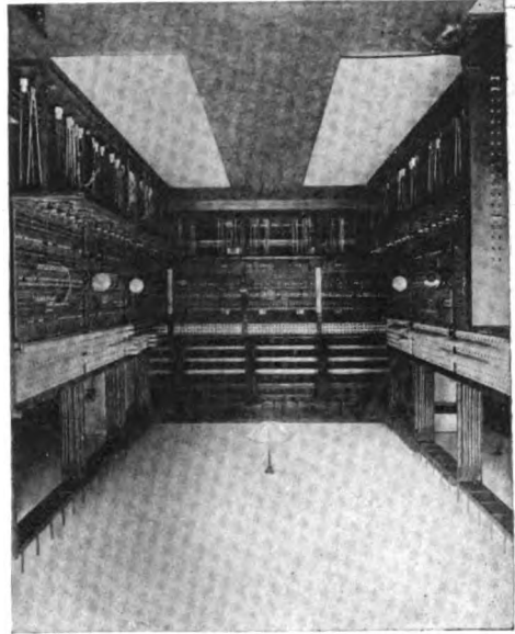
A view of one of the switchboard bays, the main line board appearing in the rear
