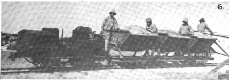
(4) One of the methods of transportation employed in delivering mast sections to the Honolulu sites. (5) Condenser pit excavations made under difficulties. (6) An illustration of the ingenuity of the Marconi engineers; the chassis of an automobile transformed into a locomotive.
